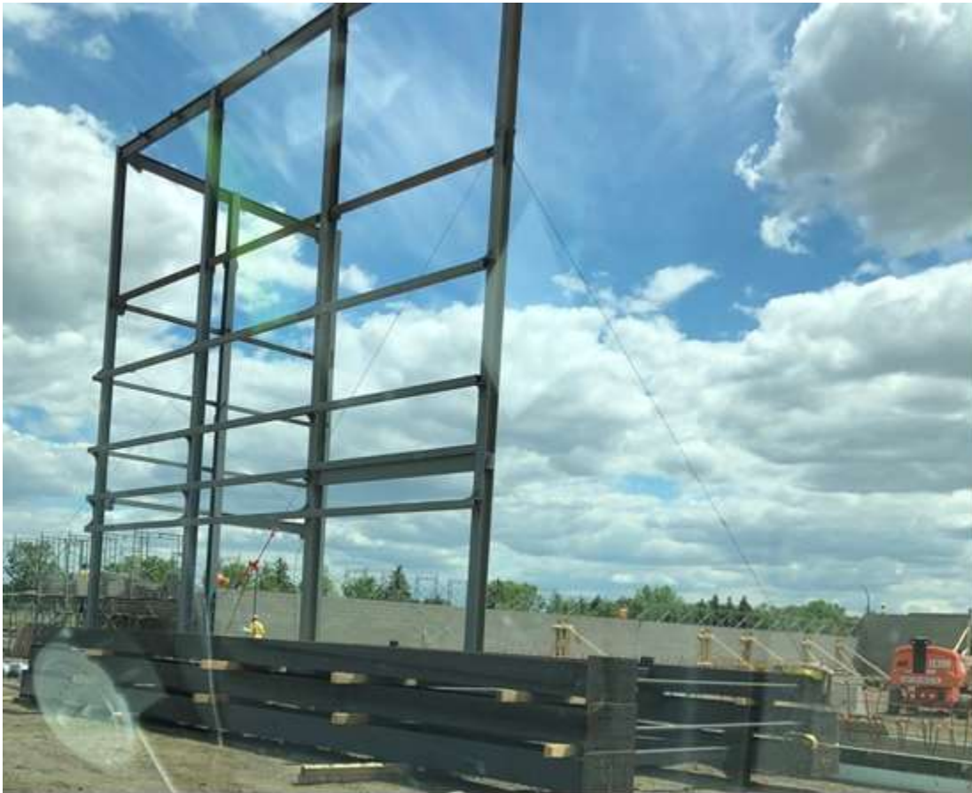
Sections 3 of 5 for one special ordered WRCC truss waiting for assembly on site.
