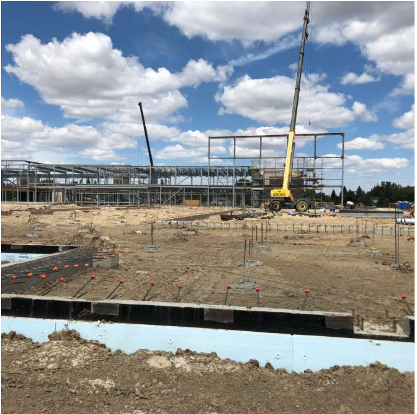
View from South end (Climb & Play Area) towards the North. Lobby, offices, arts, multipurpose rooms on left, sports turf on right.
